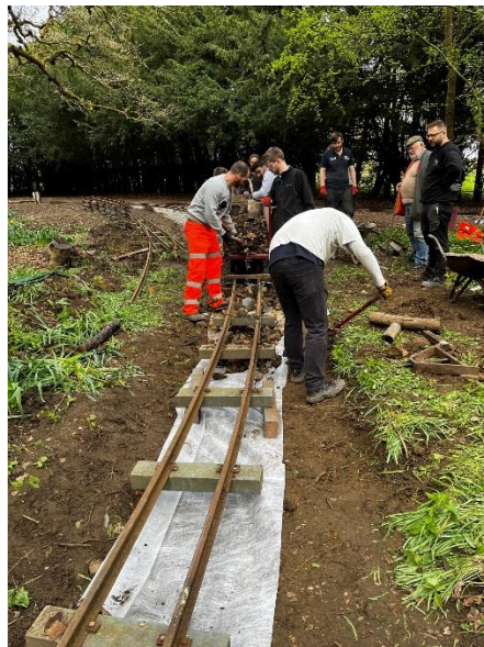
RD YMs installing the new chord linking the turntable to the existing track
